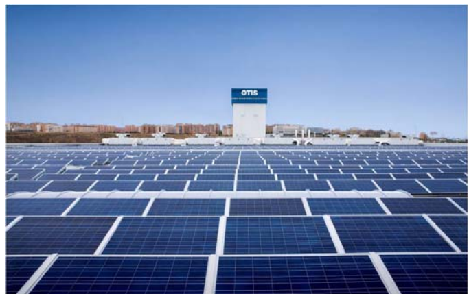
Commercial Rooftop Solar Plant
