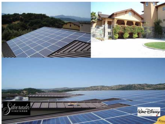
Rooftop Solar Array
